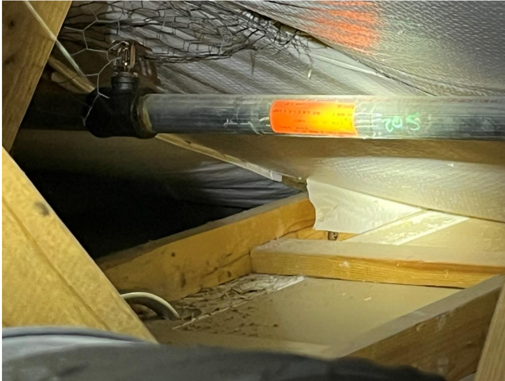
Image 6: High Roof Truss Bottom Chord Crack
