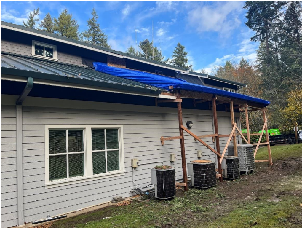
Image 5: Damaged Roof and Edge of High Roof
