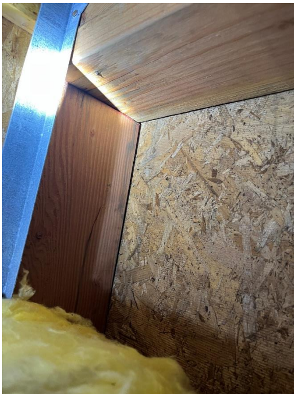
Image 9: Vertical Cracking of the Wall Stud
