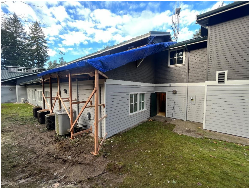
Image 1: Damaged Roof Area
