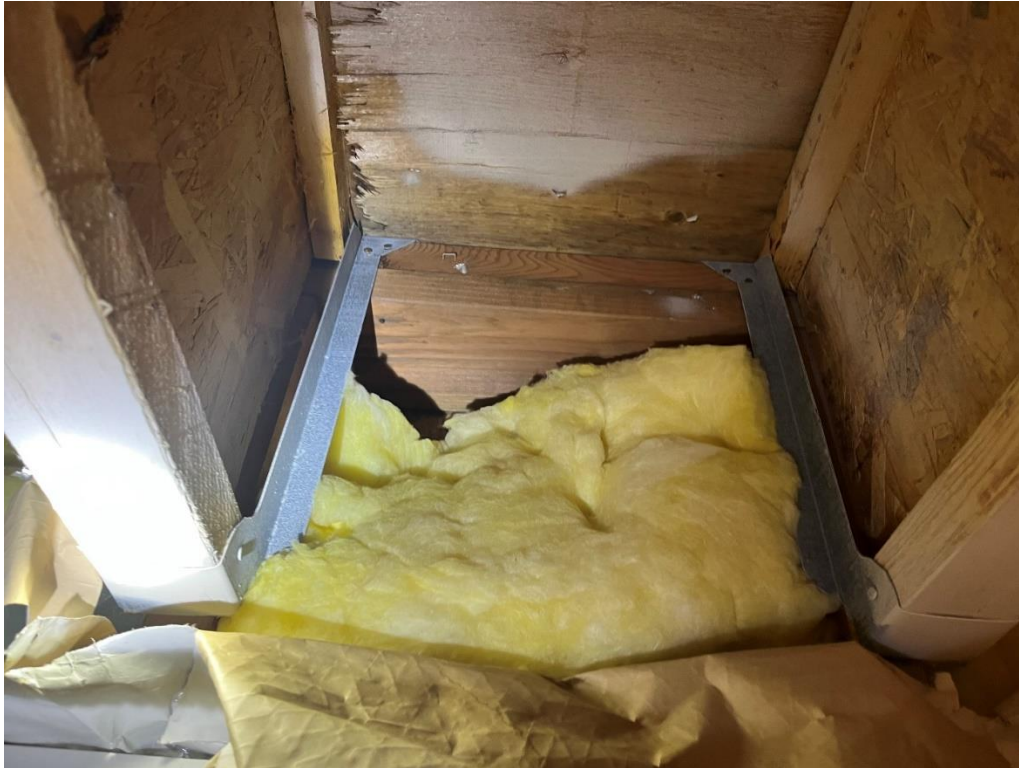
Image 8: Crushing of the Sheathing Above the I-joists
